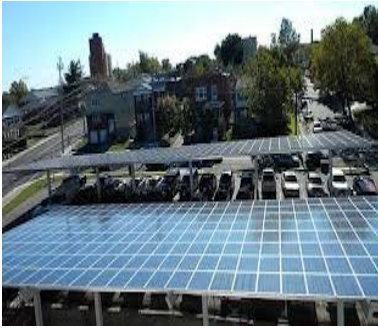
Solar panels at Secaucus Town Hall!
